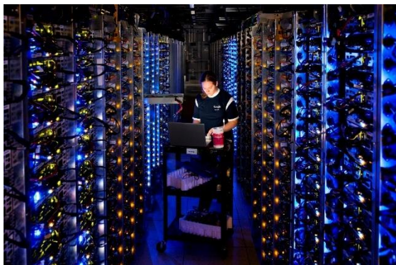
Fig. 7. Data Center Google.
